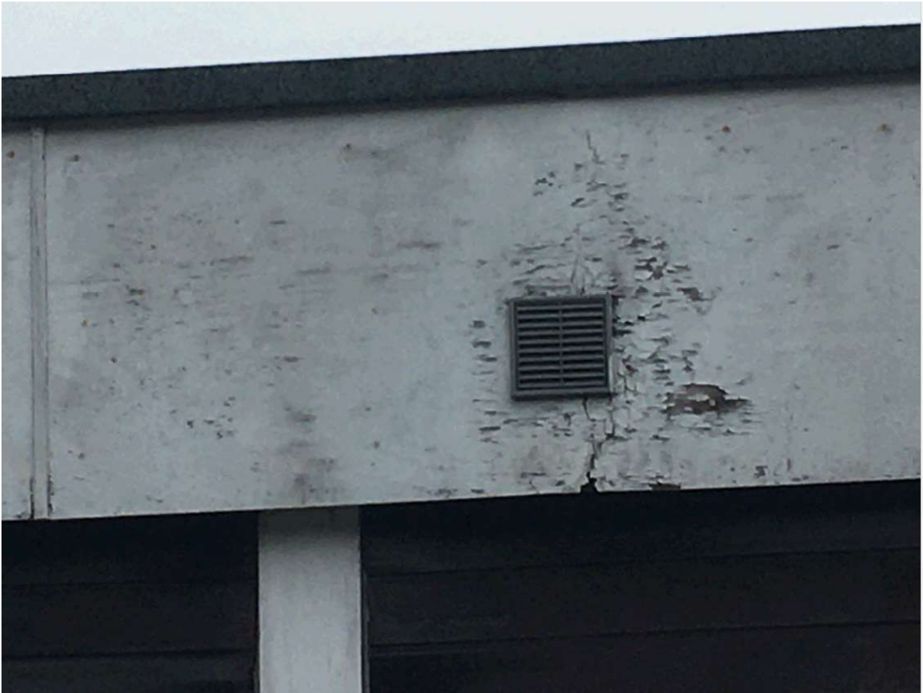
Image shows cracks to the building and its general condition
